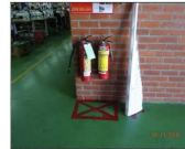
External photo(s) of the production unit(s) Fire extinguisher were well maintained.JPG
