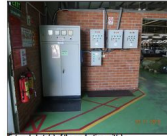
External photo(s) of the production unit(s) Fire control panel was well maintained.JPG
