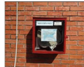
External photo(s) of the production unit(s) Fire hose reel equipped.JPG
