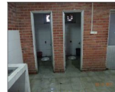
External photo(s) of the production unit(s) Fire door closed.JPG
